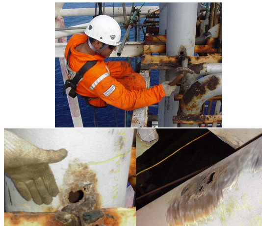
Figure 1: Corrosion damage in produced water pipelines.
