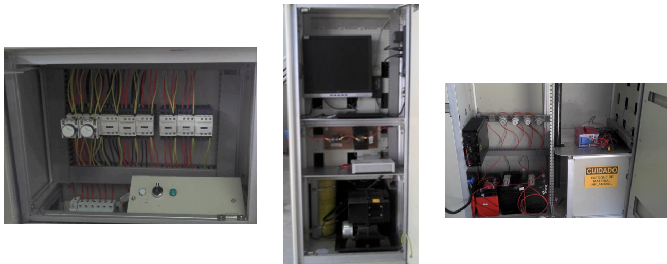
Figure 2. Manual switch (left), fuel cell control system (center), and internal view (right).
