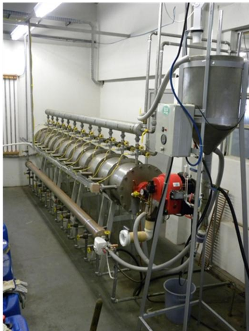
Figure 3: Furnace completely instrumented (data provided by Aymer Y. M. Cordoba).
