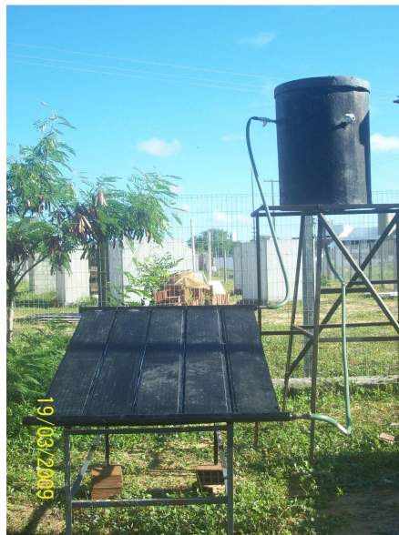
Figure 1. Water heating solar system in test.
