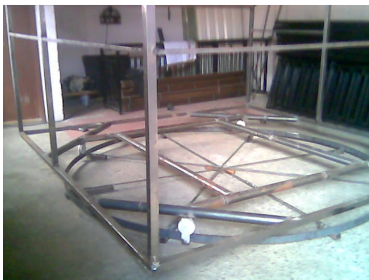
Figure 3. Details of the chamber metallic structure and its rotatory basis at the time of its construction.
