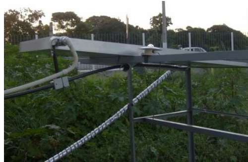
Figure 7. Solar collector and pyranometer
