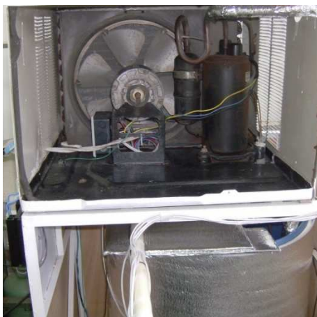
Figure 4. Compressor and reservoir
