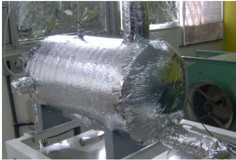
Figure 6. Boiler of the HLU
