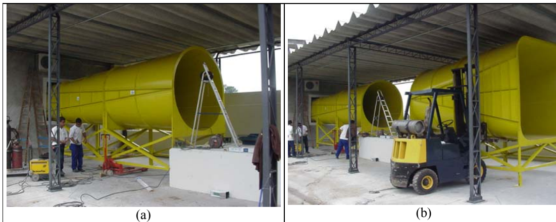
Figure 8: (a) Diffuser first part during mounting procedure and (b) Diffuser second part being positioned after the first one.
