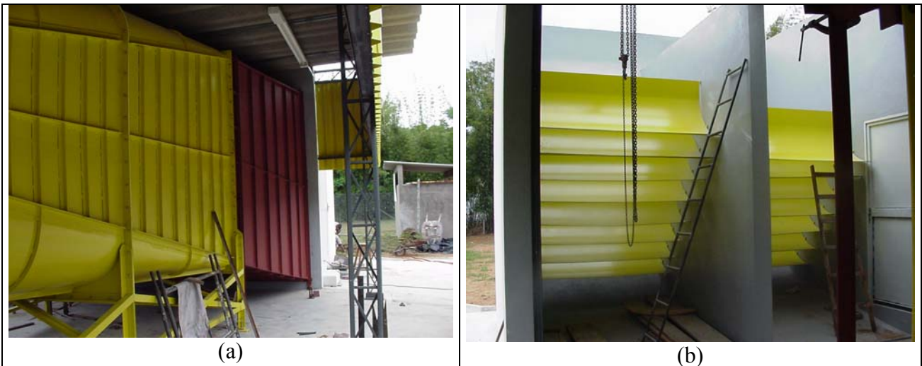
Figure 11: (a) Fast expansion diffuser (in red) (b) Internal view of the wind effect damping chamber, with vanes being installed.
